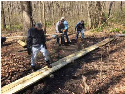
SMRA volunteers installing a puncheon boardwalk over the very muddy but heavily-used white trail at Pruyn Sanctuary. Photo: Anne Swaim
