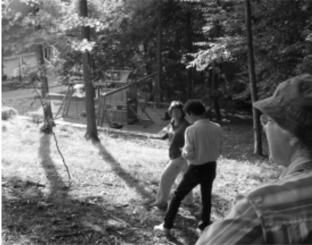
(L to R) Anne Swaim, Village Code Enforcement Officer Joe Sperber and Planning Board member Fran Allen view the damage to the Arrowcrest easement. Also present was Village Trustee Charlie Kane. Photo: Michael Madias, Jr
